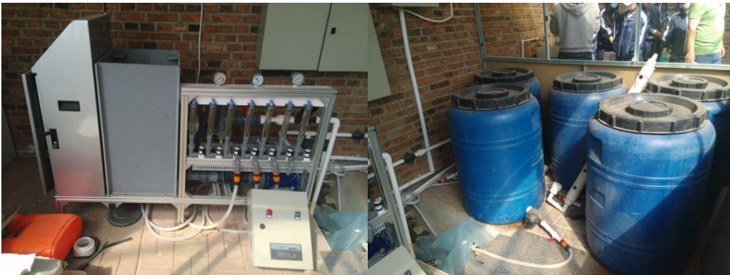
Visiting the installed MACQU system
